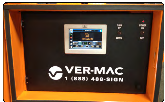
V-Touch Controller Upgrade
